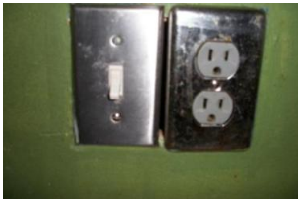
The outlet box in the kitchen is a two gang box that requires a single cover this has two single covers leaving a space between the two.
