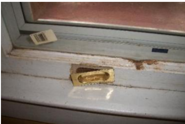
Windows are in need of repair to make them fully functional for example the ropes and weights, glass, hardware
