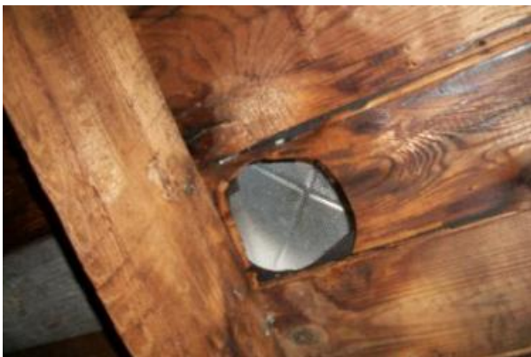
The exhaust fan vent pipe from the bathroom is disconnected in the attic
