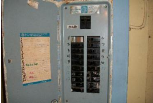
The electrical panel box is missing a blank cover plate at the number one position
