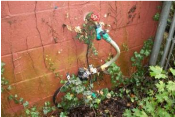
The exterior rear hose bib is leaking
