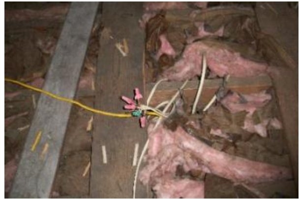
Electrical wires need to be connected inside of a junction box
