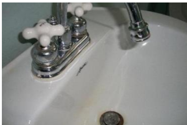
The bathroom sink faucet stopper does not function as intended
