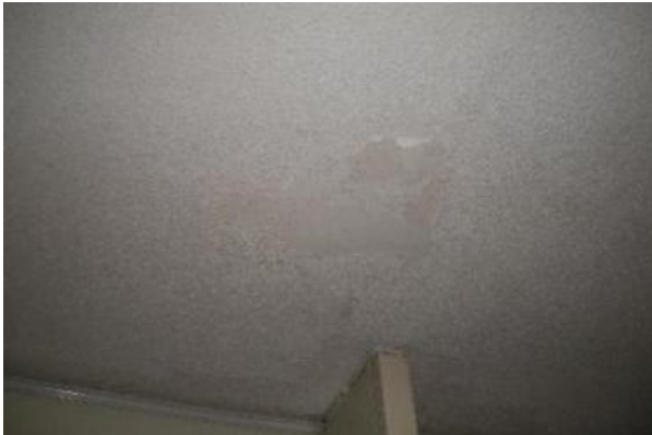
The ceiling in the kitchen shows signs of a previous water intrusion which now appears to be inactive at this time
