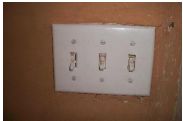
The middle switch on the living room wall operates both the ceiling fan in the living room and the ceiling fan on the front porch at the same time. Both fans are wired to the same switch
