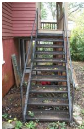
The rear porch view from the stairs side shows the slope towards the backyard
