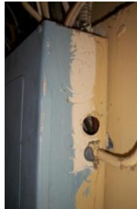
The electrical panel box is missing a cover plate at the side knockout
