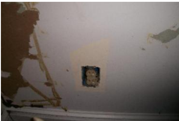
Missing cover plate
