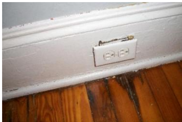
Loose Receptacle box in the front bedroom
