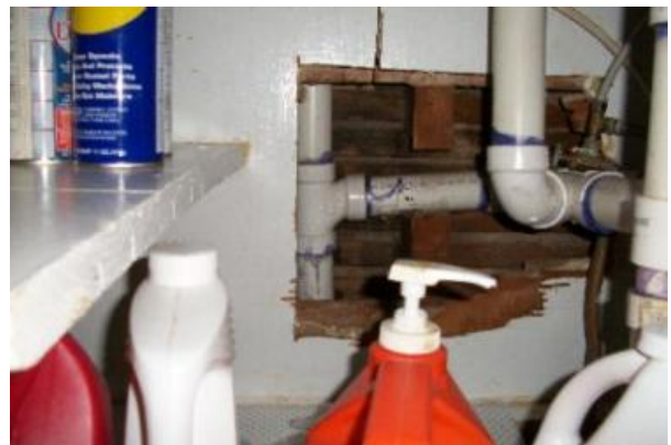
The cabinet under the kitchen sink has the back cut away exposing the interior of the wall this may have been done when there was work done to the plumbing drain system. Also this shows that the plumber has completely cut through the wall stud
