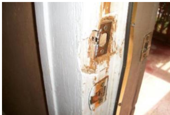
The front door jam has a lot of damage where the dead bolt secures the door.
