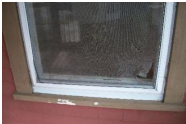
Torn window screen at the front porch
