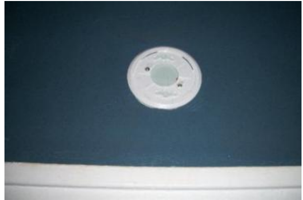
Missing smoke detector
