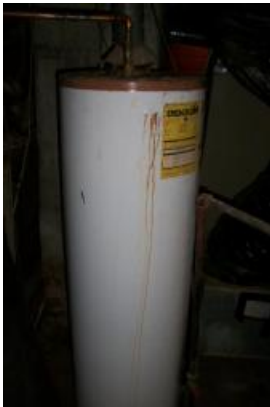
The water heater is rusting at the sides, expect to replace it in the very near future
