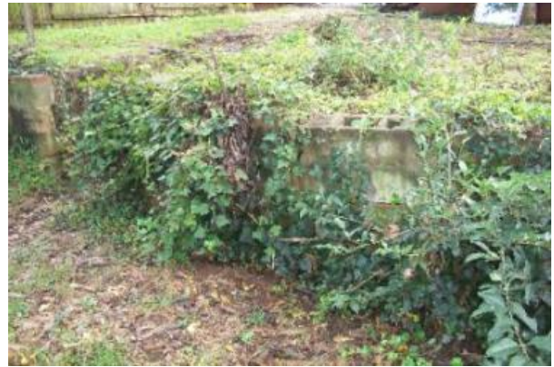
The backyard retaining wall is leaning over recommend a structural engineer evaluate.
