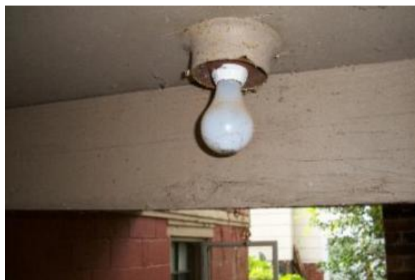
The exterior light under the back porch is missing the globe to protect the light bulb
