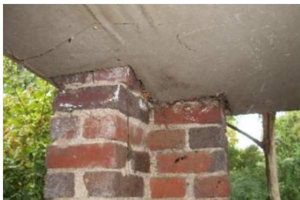
The under side of the rear porch shows signs of water damage where the boards are missing above
