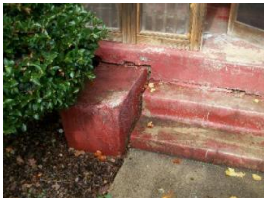
The concrete end of the front steps has settled leaving a gap between the steps and the end cap. The steps are not affected by this settlement.
