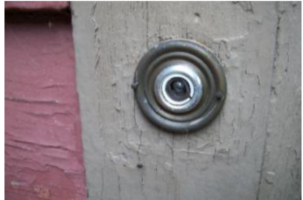
Rear door bell switch is broken
