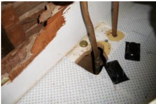
The holes under the kitchen sink need to be closed to prevent unwanted animals from entering.
