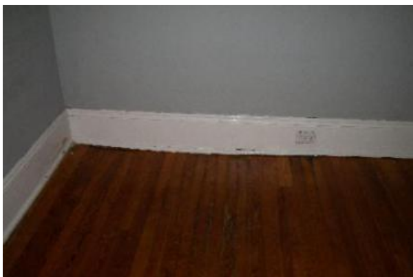
The front bedroom floor has a large dip along the common wall with the bathroom
