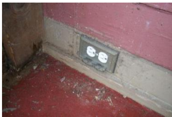
The front porch electrical receptacle is missing the weather protective cover and is not GFCI protected.
