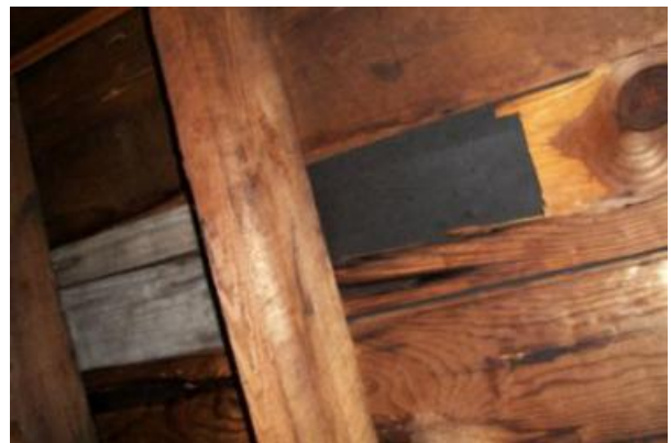
Missing roof sheathing at the left rear towards the top
