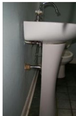
The bathroom pedestal sink is free standing
