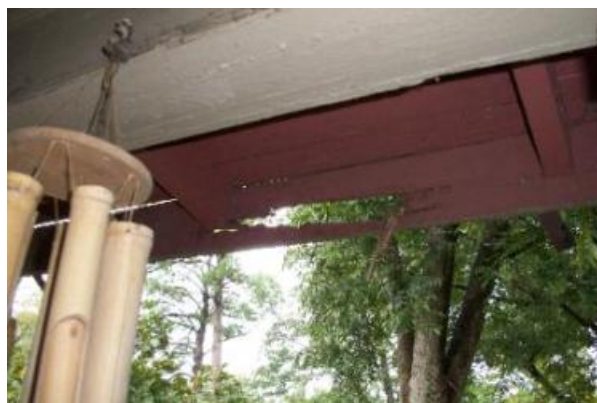
Backside view of the fascia board wood decay
