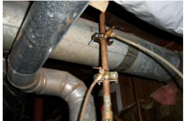
Observed saddle tap water connection that is being used for the water supply HVAC humidifier. Saddle taps are known to be problematic and to have small leaks over time. Suggest monitoring this water connection for leaks and replace with hard pipe
