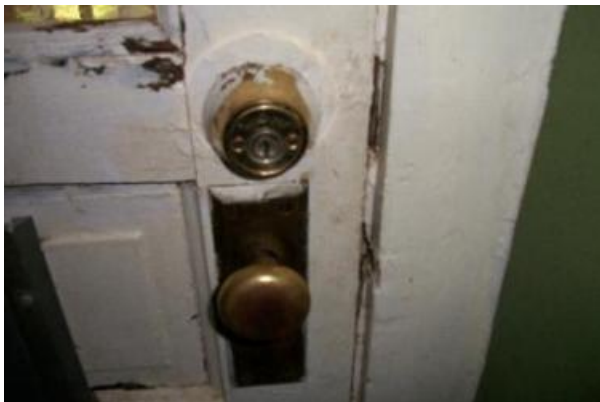
The back door from the kitchen does not latch in the closed position and there is no threshold to the door, The wood floor goes right under the door and stops 2" outside. Recommend replacement of the door by a professional contractor
