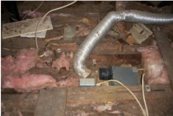
The exhaust fan vent pipe from the bathroom is disconnected in the attic
