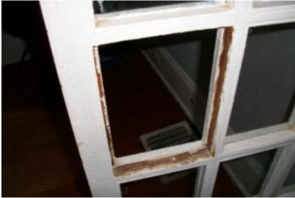
Missing Glass between the Living and Dining rooms
