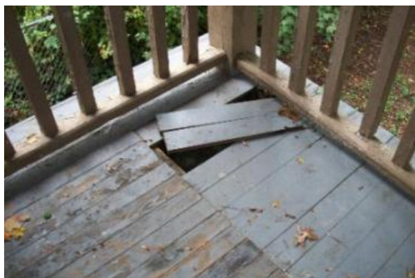
The rear elevated porch has wood damage and loose or missing boards as well as a low railing and the flooring of the porch is sloping downward towards the backyard. Recommend a General contractor or a Structural Engineer evaluate the rear porch.
