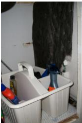
The is no cabinet wall between the dishwasher and the kitchen sink. This can allow for items places in the cabinet to fall into the dishwasher area and make their retrieval very difficult
