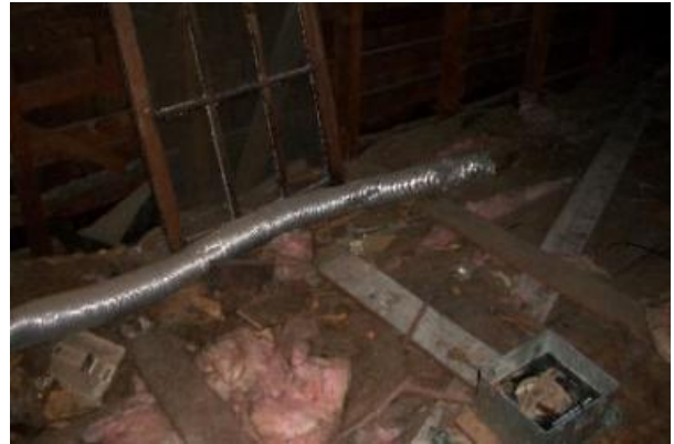
The exhaust fan vent pipe from the bathroom is disconnected in the attic
