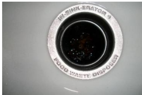
Splash guard that protects operator from contents being through from the appliance during operation located in the throat of the sink drain is deteriorated and needs to be replaced.
